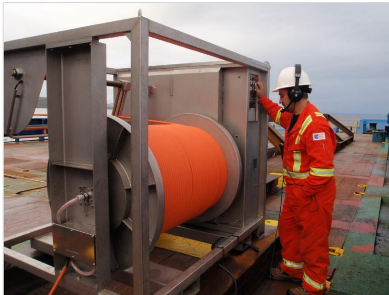
Figure 10 – AC umbilical winch.
