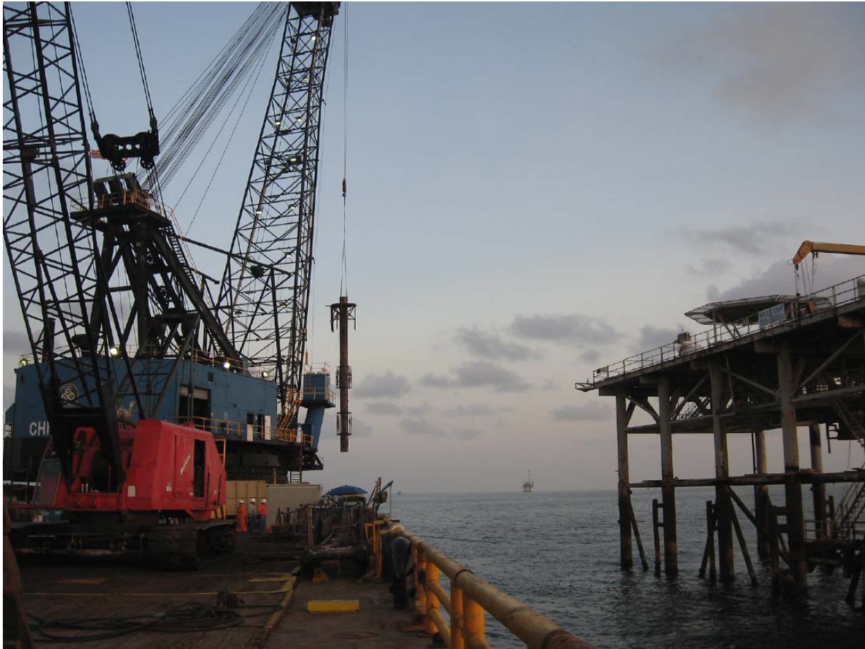
Photo#1: Structure Maritech F4 Complex ID 20887-1 at Right with Diver-Cut Caisson F (Complex ID 20887-2) Being Pulled
