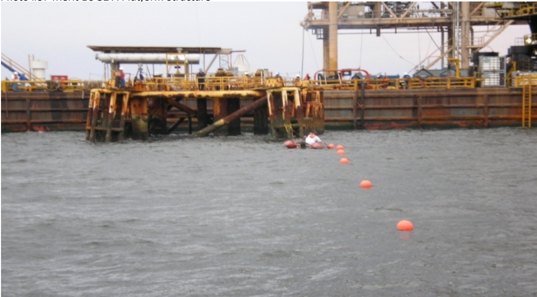
Photo #10: Merit EC-32A platform structure showing acoustic shock measurement array deployment.
