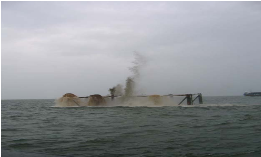
Photo #8: Delay shot sequence on piles A1 through A5 and B1 through B5 and conductor F3
