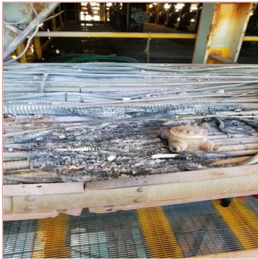
Damaged Area from Fire.
