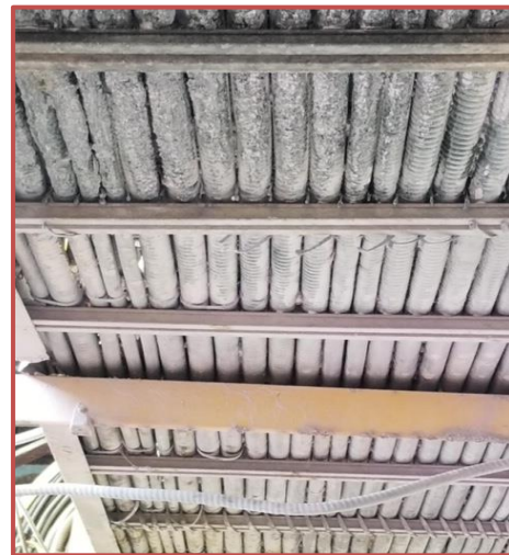
Bottom-view of Cable Damage.
