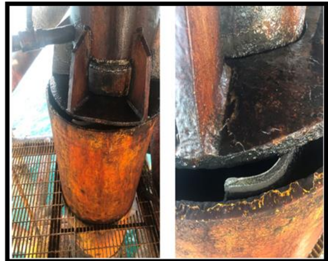
Figure 2 - Part of casing protruding out of well drive-pipe.
