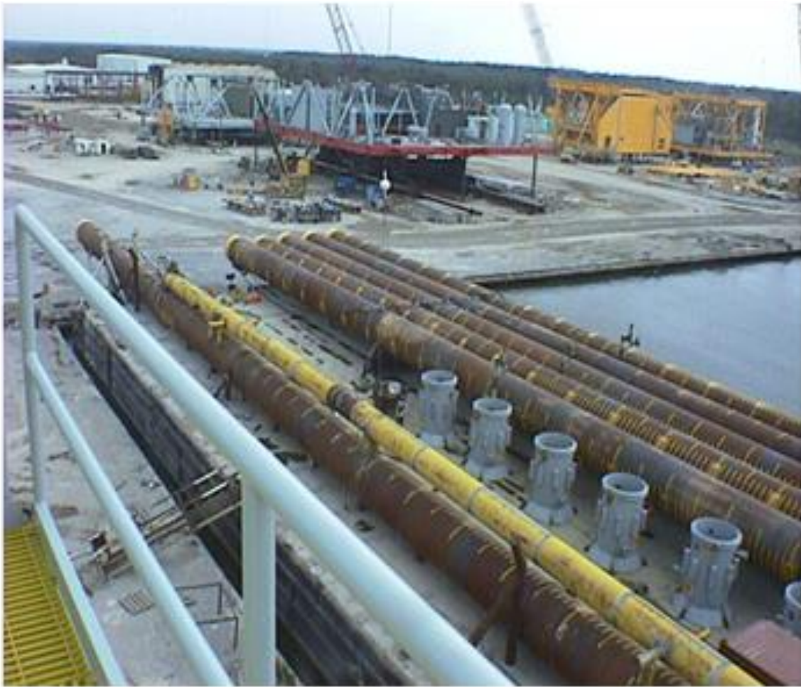
Figure 2.6 - Piles with receptacles attached. The CP anode sleeves shown are installed after pile driving. (Photo courtesy of ENI)
