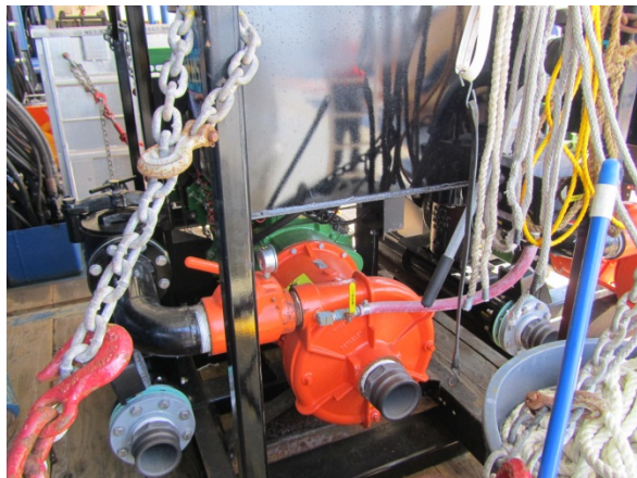
Fire Boom Power Pack
