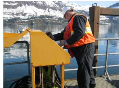
LSC-5 Control Panel
