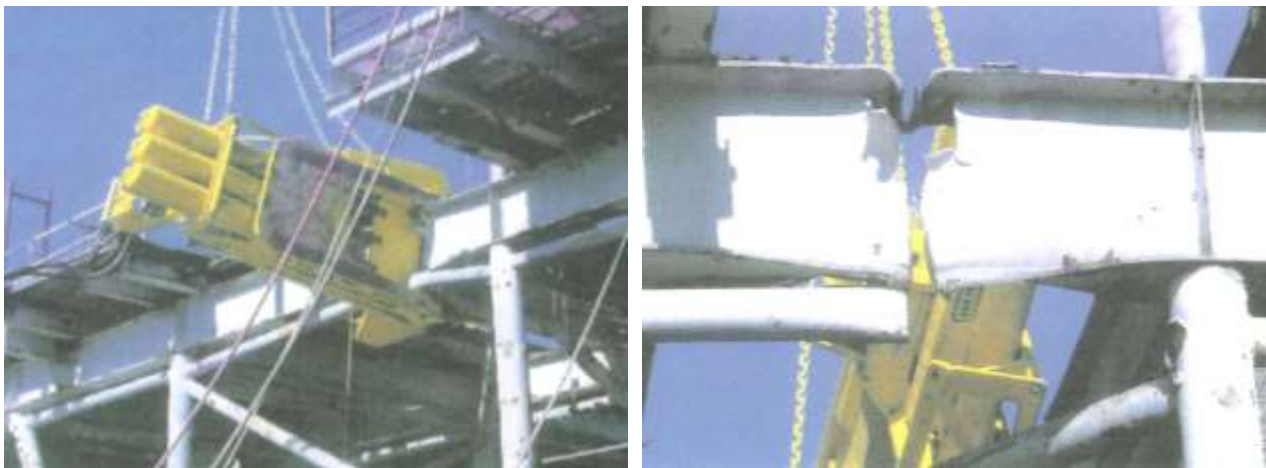
Figure 6-26. Power Shear Cutting Platform Deck Beam (Photo courtesy of Prime Marine Services, Inc.)
