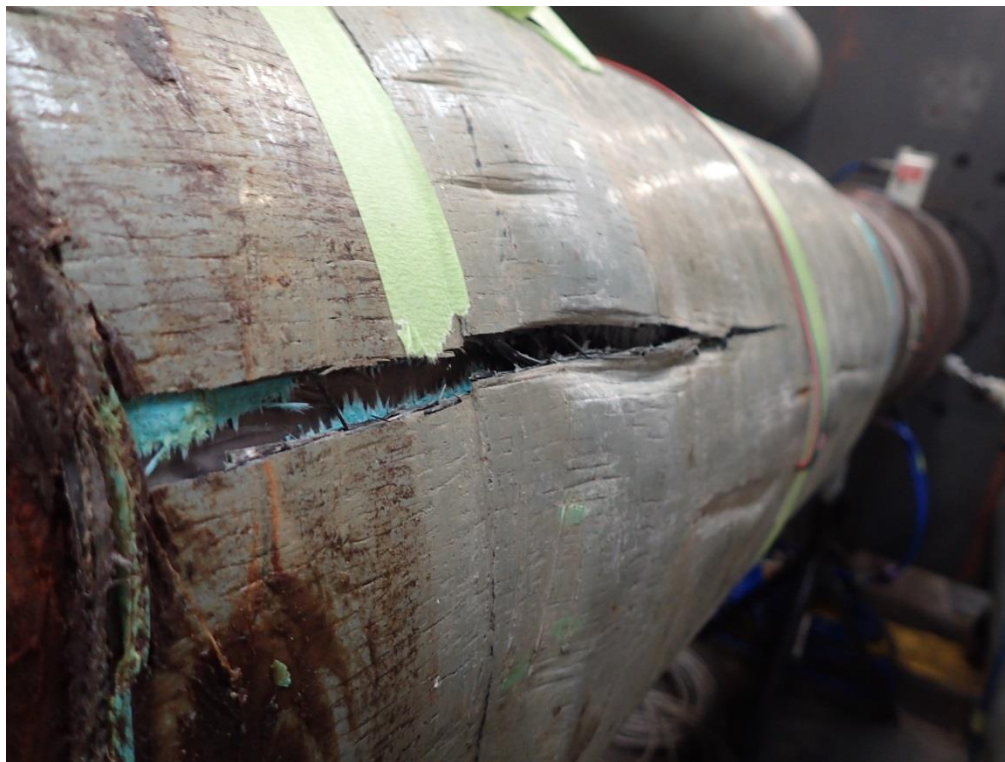
Figure 5-20: Manufacturer C’s delamination sample (OFF-C-DL-J3-5) post test with large crack in composite repair
