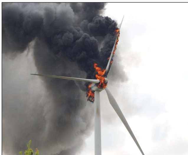
Figure 2 – Windpark Groß Eilstorf wind turbine fire [8]
