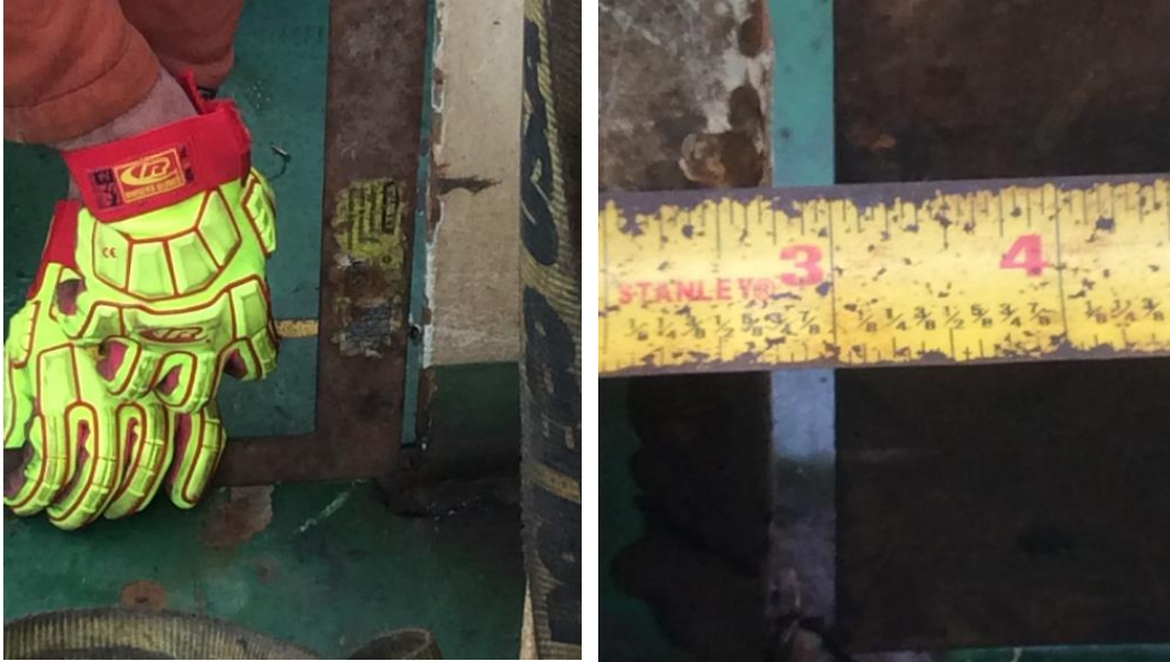
Figure 12 - Out of square measurement
