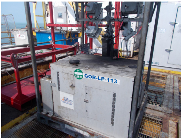
Figure 1: Rental generator/light plant.
