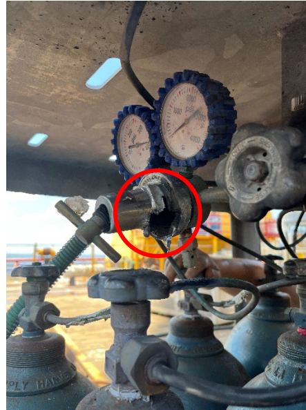
Figure 2: Damage to aluminum fitting on regulator.
