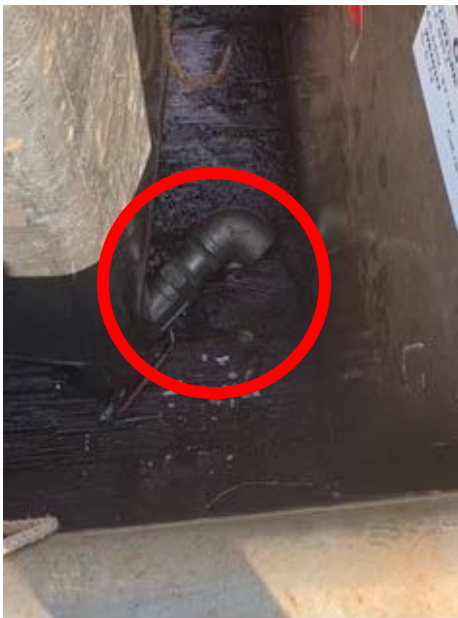
Figure 1: Tote tank drain nozzle separated from tank after impact with another object, resulting in loss of containment.
