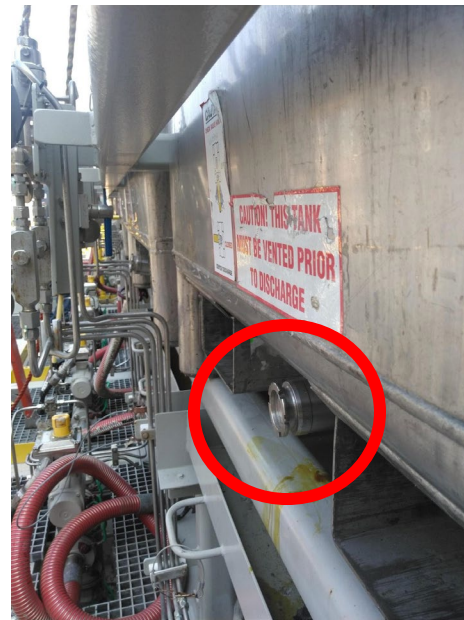
Figure 2: Tote tank drain nozzle cracked after contact with rack, resulting in a leak.
