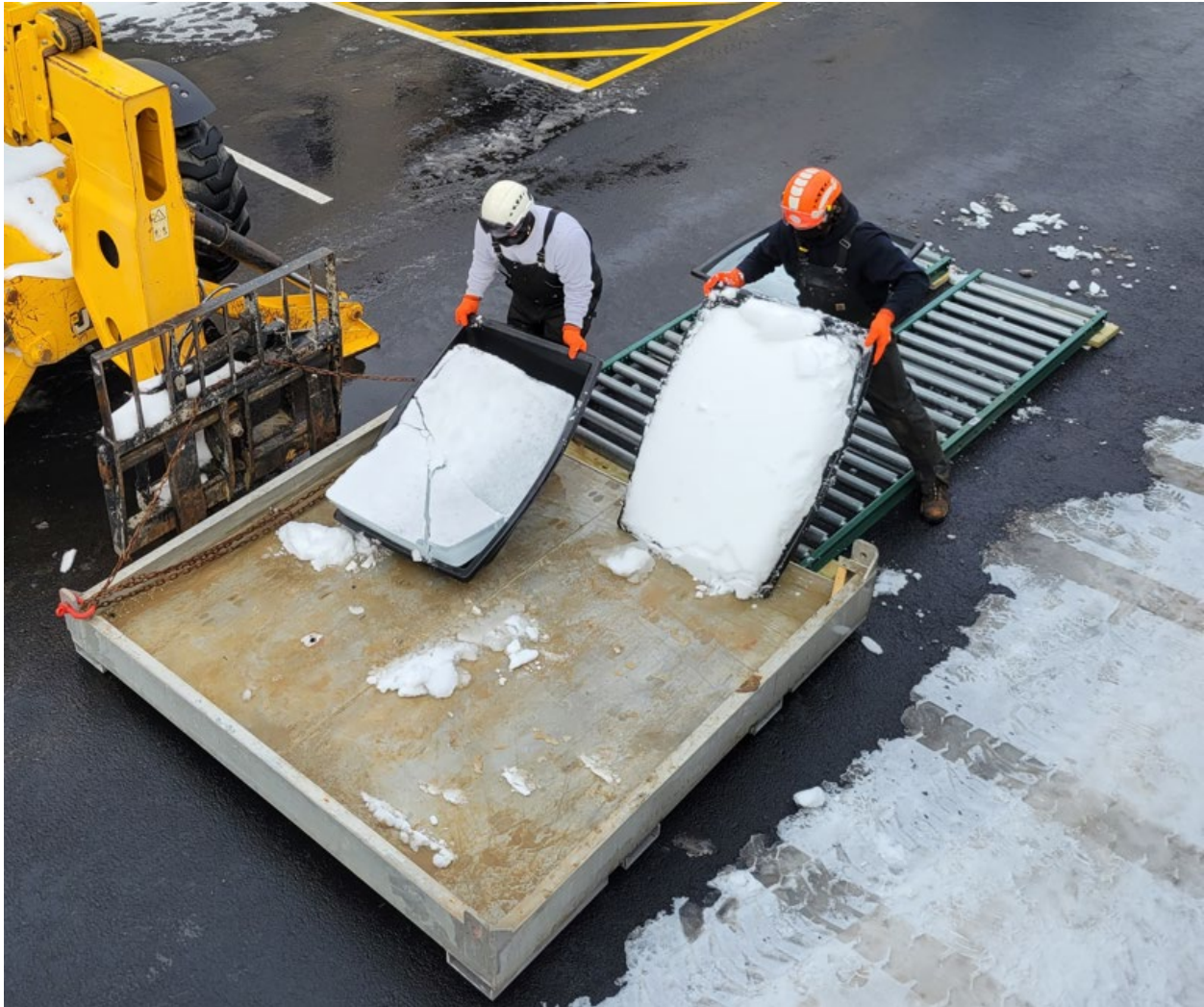
Fig. 3 Ice blocks slide out of the plastic mortar bins as they are rotated vertically
