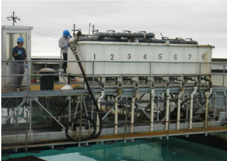
Fig. 4 Auxiliary Bridge Recovery Tanks
