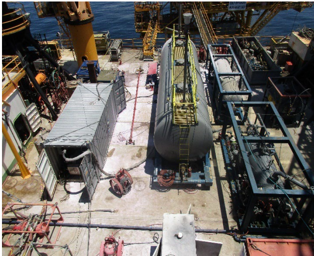
Figure 1. Test separator and 500-barrel tank.
