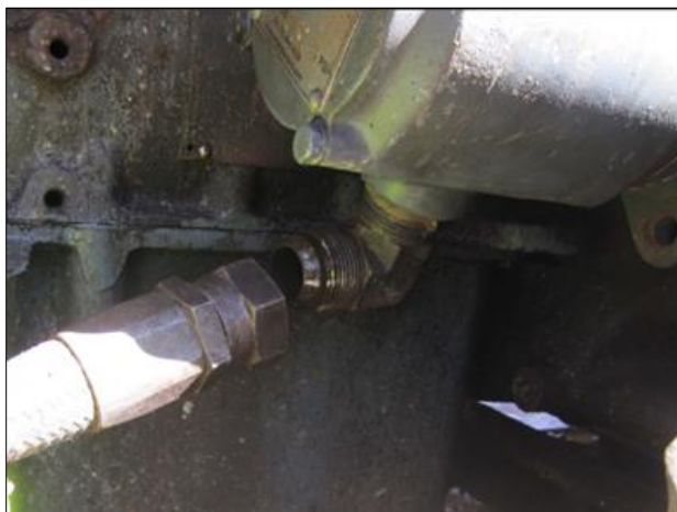
Figure 1: Gas starter vent line, shown post incident, was only partially connected. (Incident 1)
