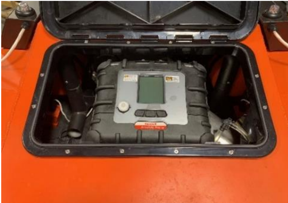
Fig. 10 Gas detection system
