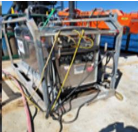
Figure 1-Small Flames on Left Side of Plug during Welding Operations
