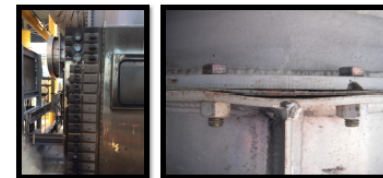
Burn Damage (left), and the Gap in the Mating Flange in One of the Fire Tubes (right)
