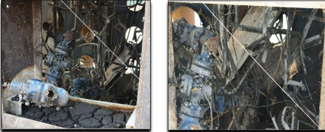
Figure 22. Post Incident Condition of MC 20 Wells
