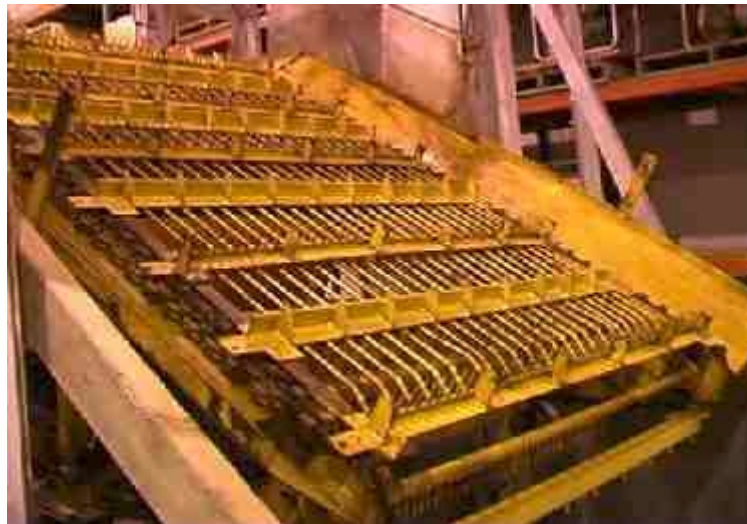
Figure 3.5 Lifting Grated Belt installed on work platform. New rakes have been added in between old ones.
