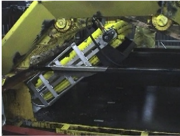
Figure 3.11 LORI Brush Pack installed backwards in LGB, Hamburg. Operational direction is to the right.
