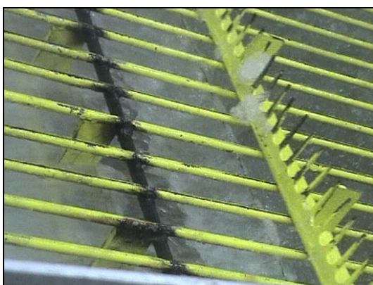
After modification. Two of every three pieces of flat iron supporting the grating bars have been removed. To support the bars, a thicker cross bar (black) has been welded to the grating.
