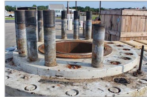
Figure 4: Hydraulic connector flange/fasteners showing failures and first engaged threads
