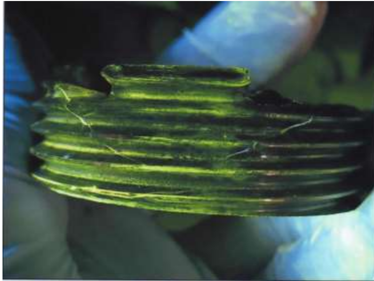
FIGURE 6: CRACKS PROPOGATION THAT EXTEND INTO THE THREADS BELOW THE FRACTURE FACE INTO THE THREADS (OEM RCA)
