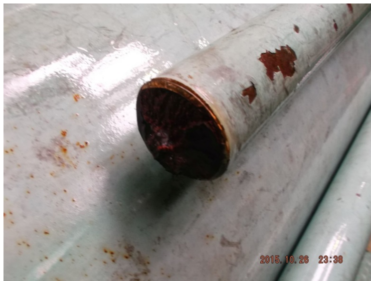
FIGURE 8: UPPER BSR FASTENER FAILURES – CLOSE-UP OF FRACTURED FASTENER
