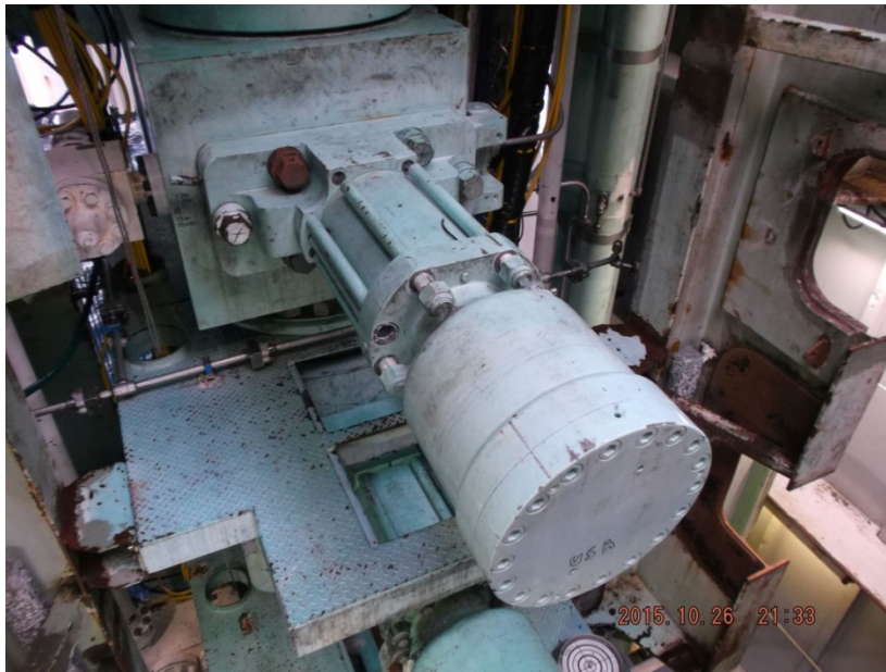
FIGURE 5: UPPER BSR FASTENER FAILURES
