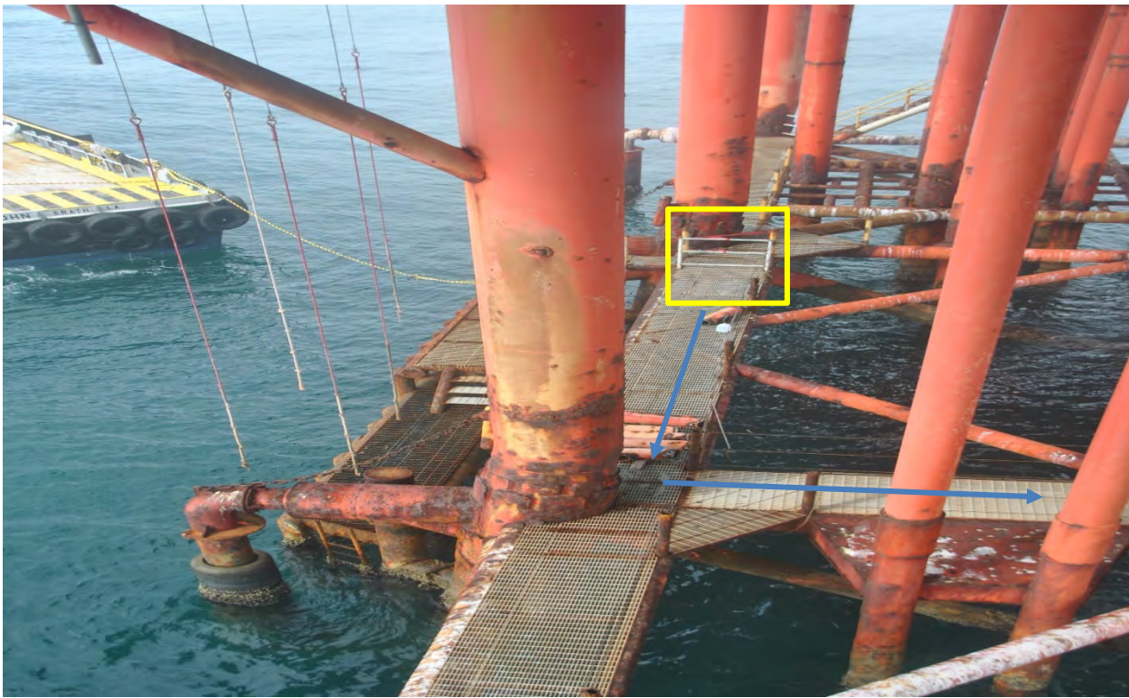
Figure 8: Barricade blocking access to out of service area where the landing zone / storage area were established. (Arrows show area designated as out of service)
