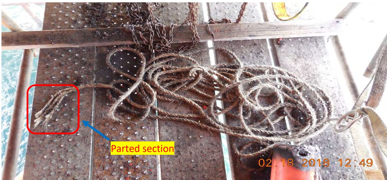
Figure 12: ½-inch manila rope that parted during firewater piping removal.
