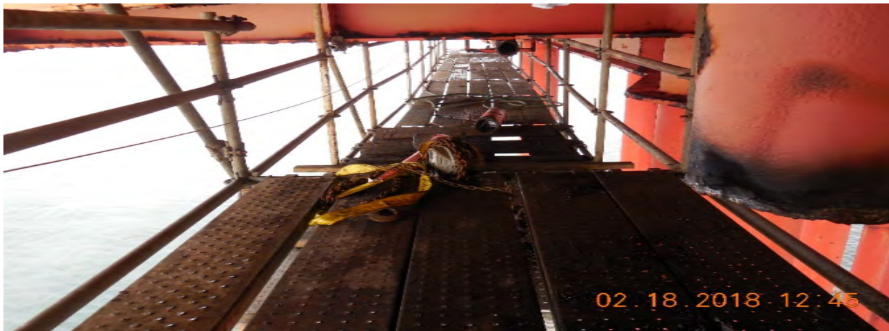
Figure 6: West side scaffolding without toe boards and visual of accommodation to lower scaffolding.
