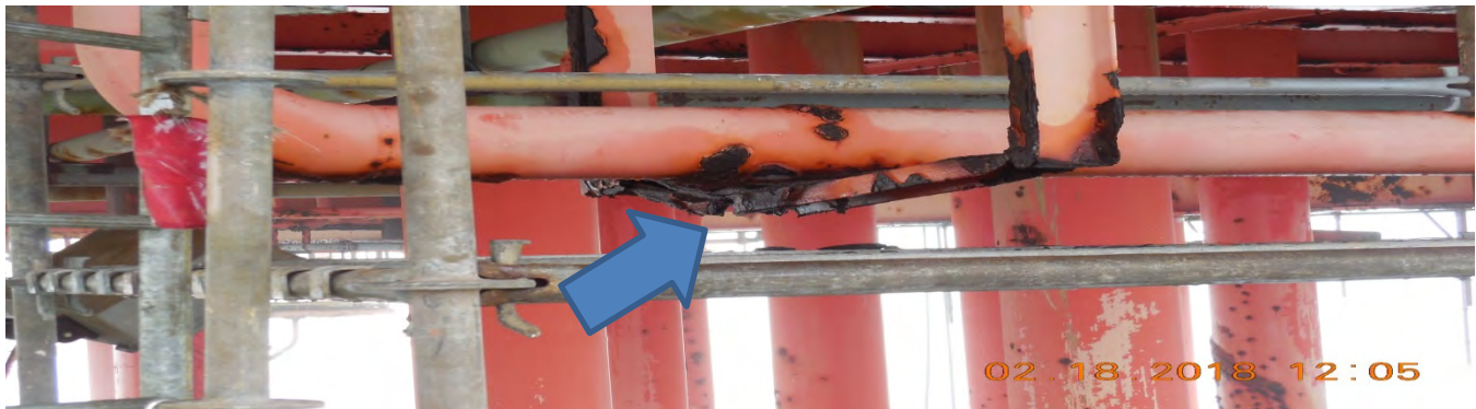
Figure 3: Rusted firewater piping support bracket
