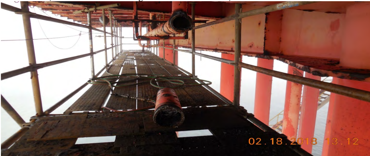
Figure 9: Distance where construction workers allowed pipe to fall to scaffolding deck.
