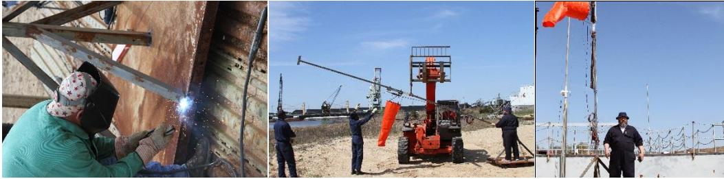
Figure 65: OGES tower assembly and raising: A base was welded to support the 7 meter tower (left) then raised via forklift (center) and instrumented (left).
