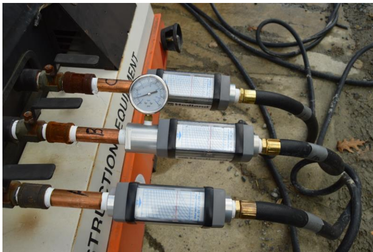
Figure 20: Hedland Air Flow rotameters mounted on air compressor.
