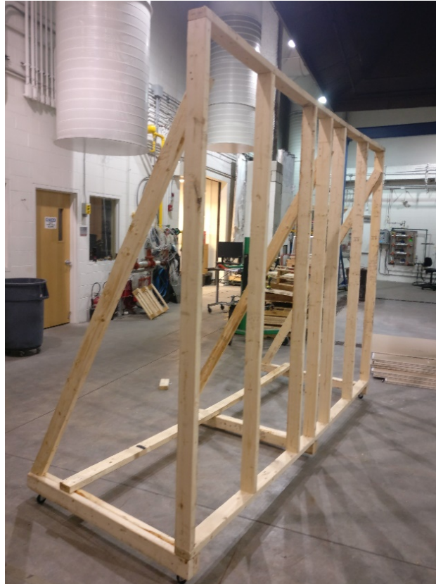
Figure A1. Lumber frame for holding sheetrock boards. Lumber cross-section were (2" x 4").
