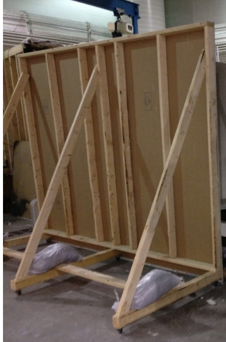
Figure A2. Sheetrock installed on the lumber frame. The side visible was on the outside of the fire whirl enclosure.
