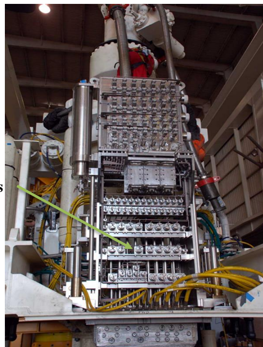
Figure 2: Example of SPMs Mounted Horizontally within a Control Pod
