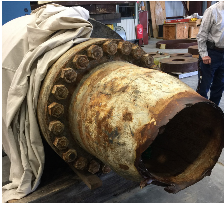
Failed Riser Adapter
