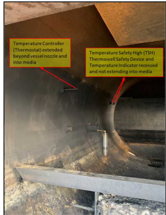
The TSH is not extended far enough into the heat media. As a result, the Temperature Indicator (TI) is unable to register a proper temperature.
