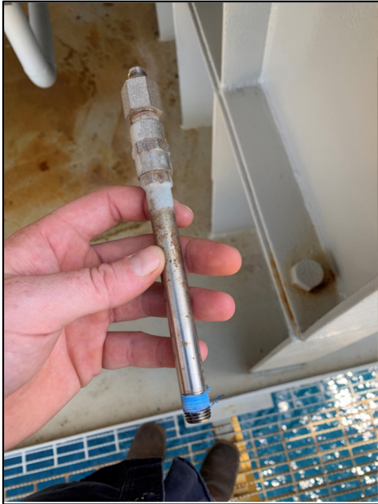
A Temperature Safety High (TSH) with Teflon tape on the threads. Teflon tape reduces the heat sink effect.
