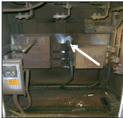
Short circuit fault in the ASD
