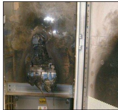
Arc damage to components
