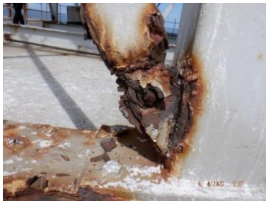
Figure 1 - Helideck structural support bracings in poor condition
