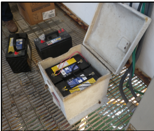
A typical battery enclosure is shown above. The service start dates have been written on the batteries.
