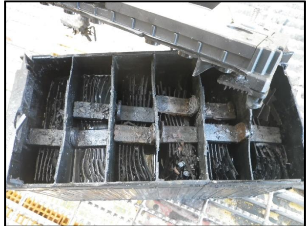
This battery may have exploded because it was charged with a second battery that had a malfunction, causing this battery to overcharge.
