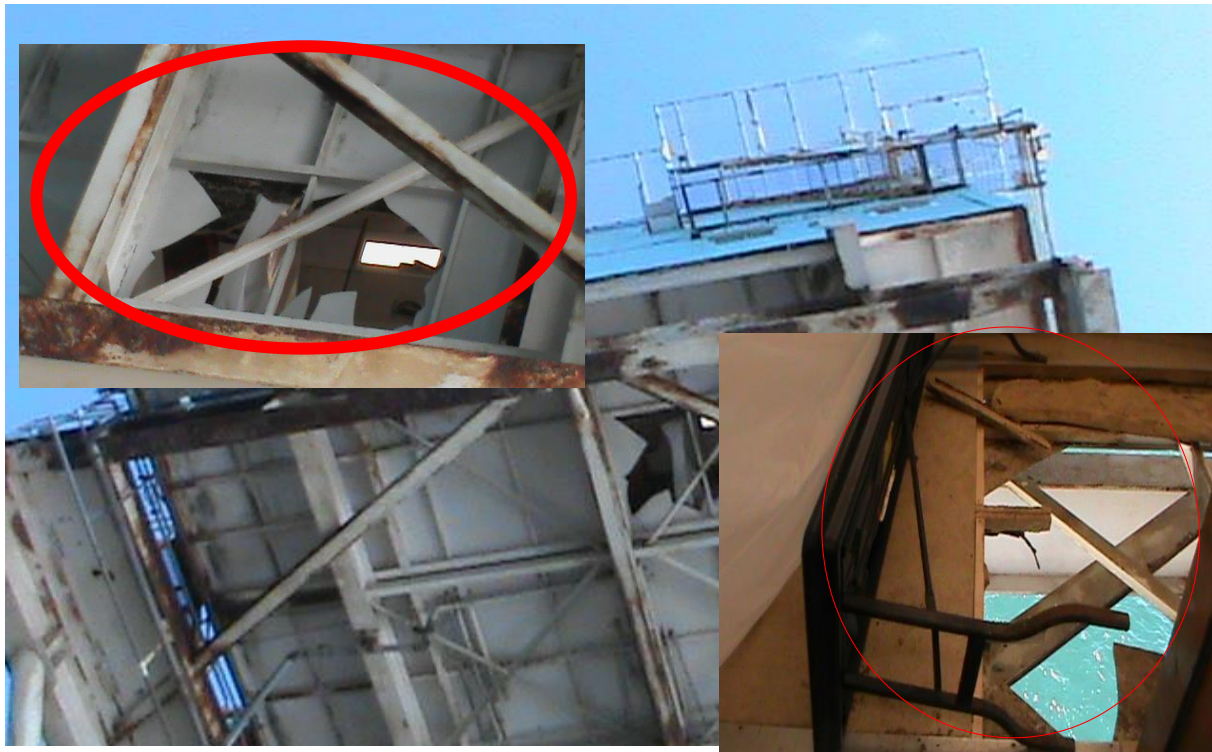
Images of the shattered floor material
