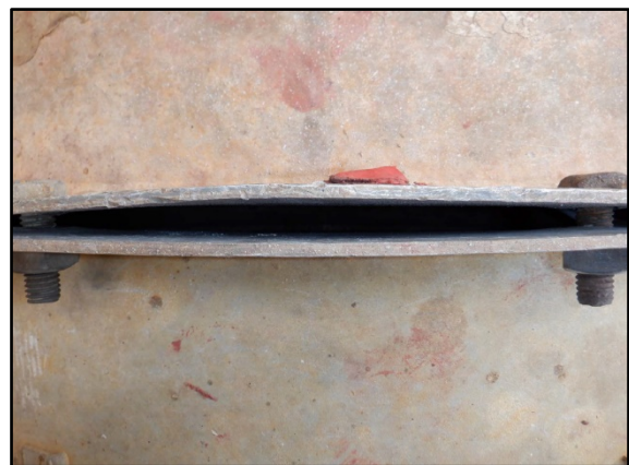
A gap in a Heater Treater flange is shown with no Gasket
