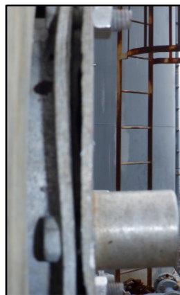
A warped Reboiler flange
