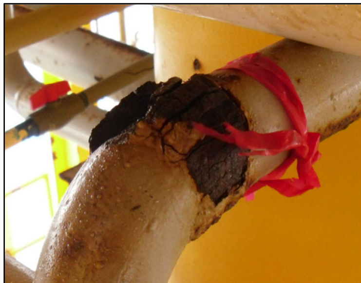
A leak was found in this 2" vent line during compressor blow down.
