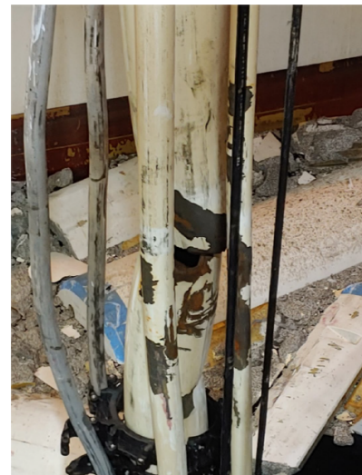
Figure 2: Ruptured Riser Joint
