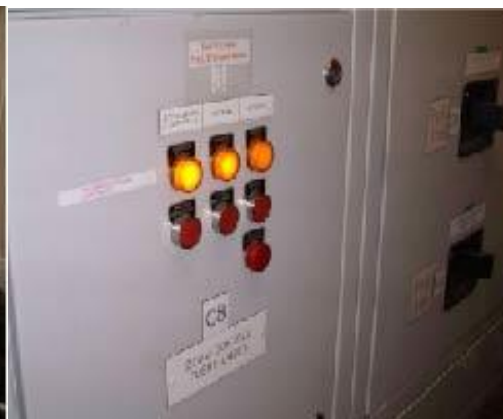
Figure 2 - Switchboard open/reset command buttons
