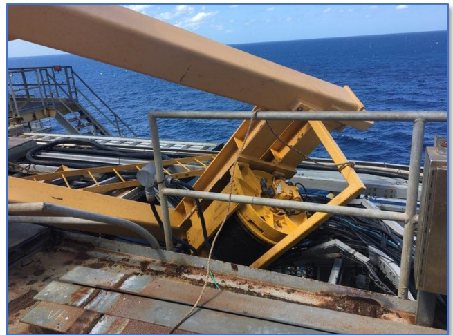
Figure 2. Gantry Contacting and Damaging the Cable Tray and Bending the Main Deck Handrail
