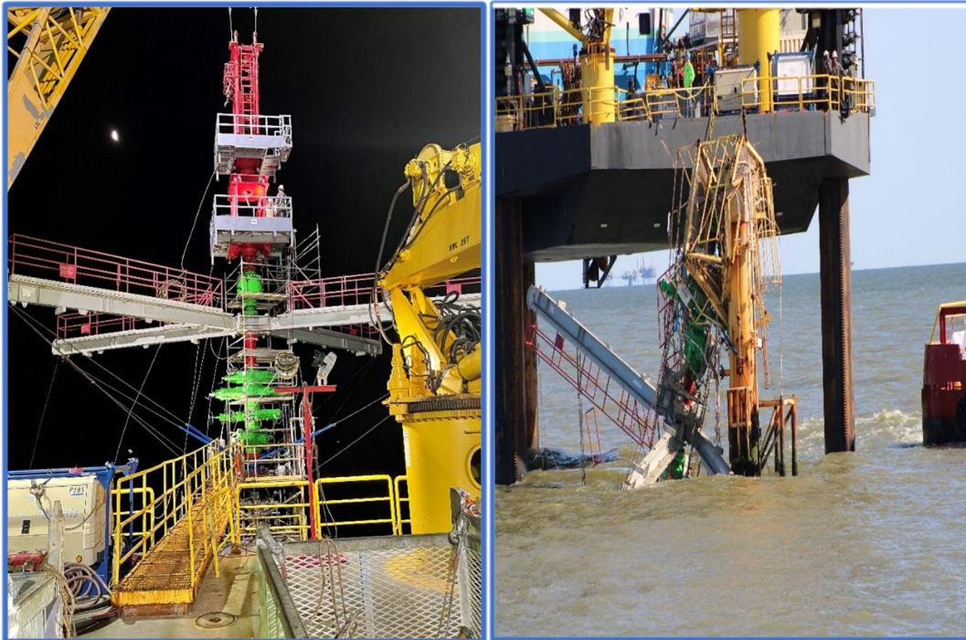
Hydraulic Workover Unit Before(left) and After (right) Fatal Incident
