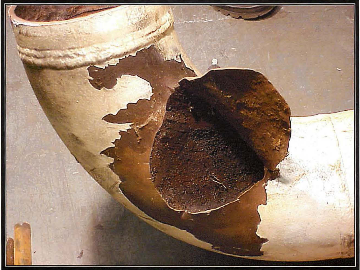
Appendix A.6-Ruptured Elbow
