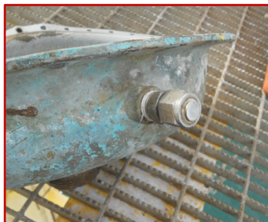
Capped off fitting in place of pressure relief device
