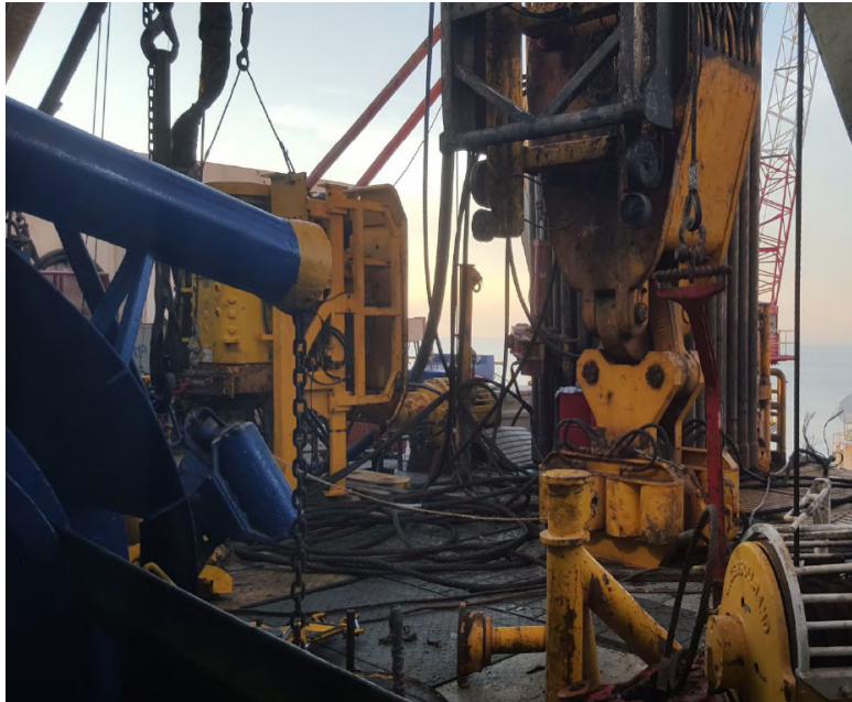
View of traveling block and unspooled cable drill line on rig floor following the July 20, 2017 incident.
