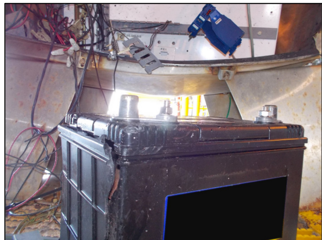
Overcharged 12 Volt Battery
