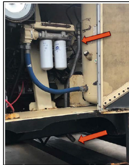
Photo 2 – Relief Line Leading to Skid
