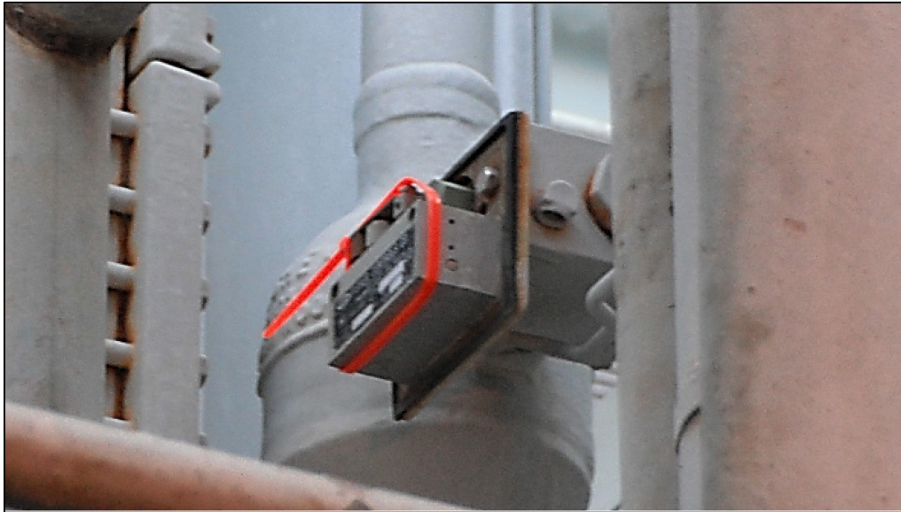
A level safety high deactivated with a zip tie.
