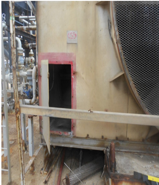
Figure 1. Access hatch for compressor cooling fan
