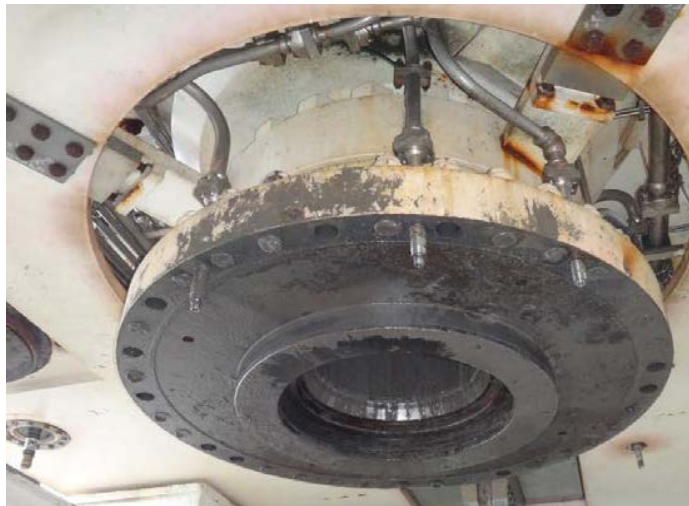
Upper half of failed LMRP Connector
